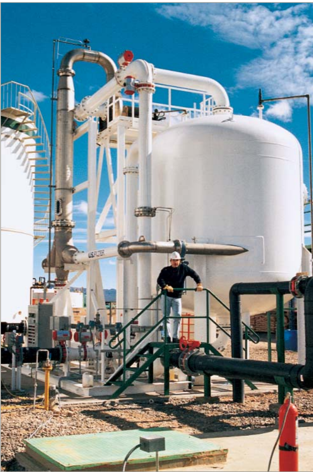
Figure 2. Tertiary produced water separation treatment methods include walnut shell, media, cartridge and activated carbon filtration.
