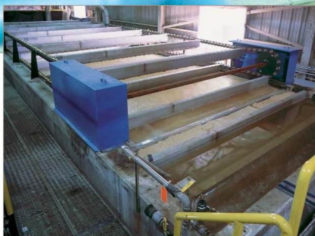
Figure 3. In DAF separators, influent is mixed with countless micron sized air bubbles as the flow enters the tank.
