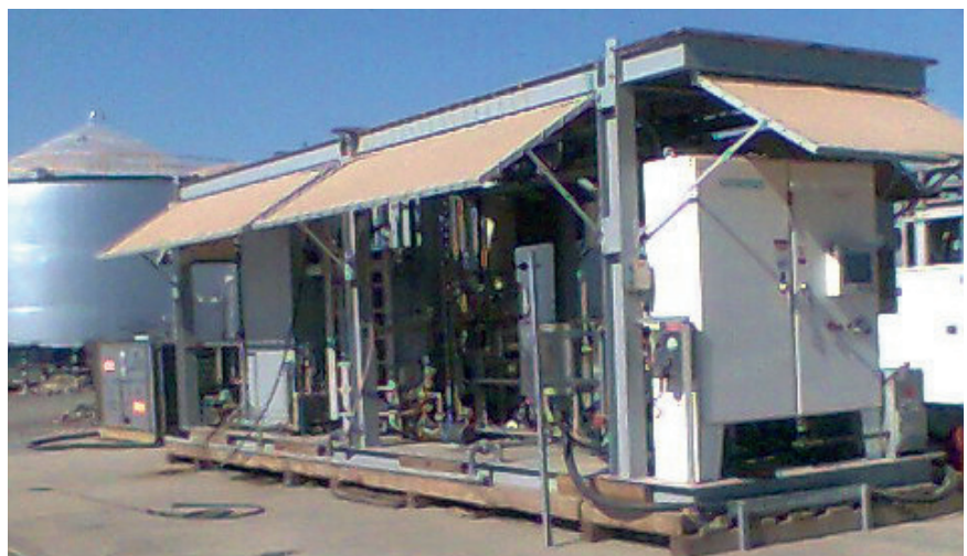
EcoRight® pilot unit in operation at a Saudi Aramco Refinery
